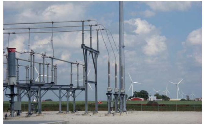
Twin Groves Phase I Substation
