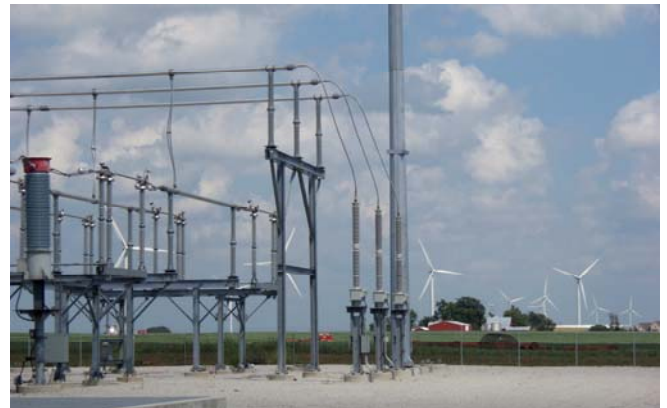
Twin Groves Phase I Substation
