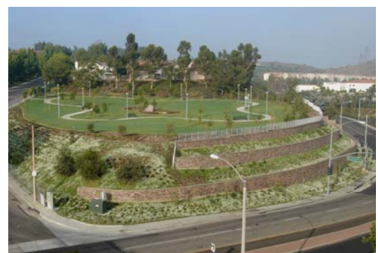
Roosevelt Park Conceals the Completed Park Substation
