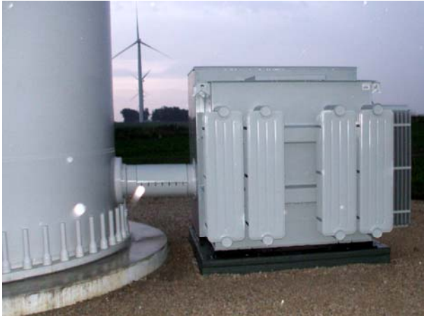
34.5-kV/600-V Collection System Pad-mount
