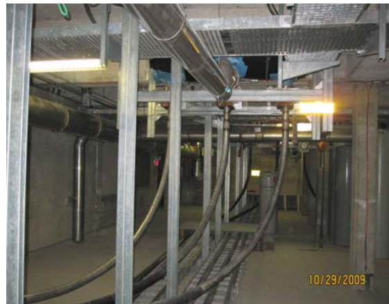
Existing Substation Cable Vault
