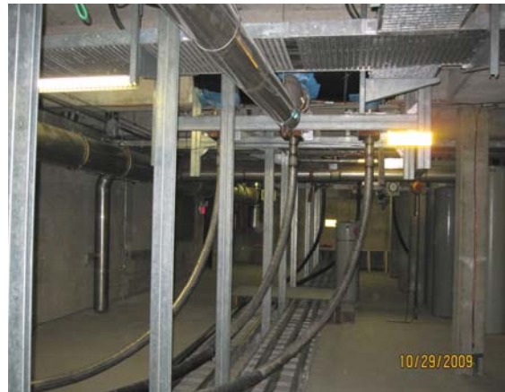
Existing Substation Cable Vault
