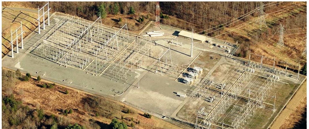
Brighton Substation Prior to Expansion
