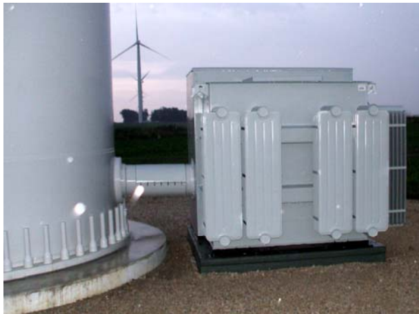
34.5-kV/600-V Collection System Pad-mount
