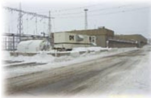
Bruce A Nuclear's temporary qualified power supply (QPS). Photo courtesy of ASLF.
